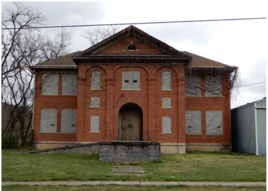
Front elevation showing added loading dock, boarded up front door, blocked windows with small vents and invasive vines in cornice and roof.
