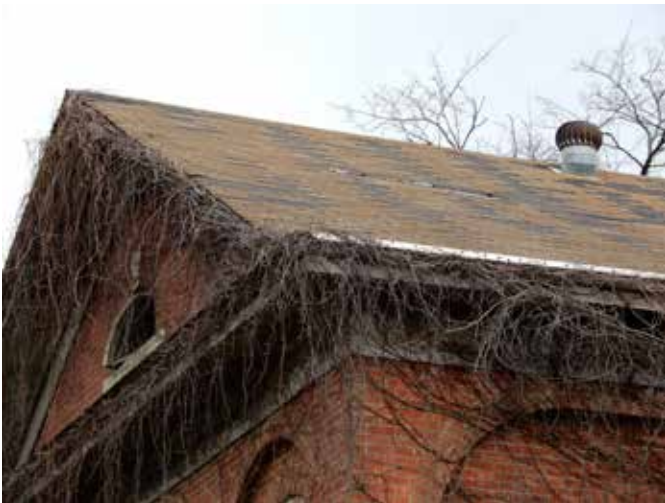
View of deteriorated asphalt shingle roof and invasive vines at roof cornice.
