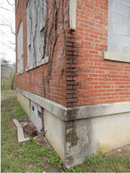
View of mortar damage due to lack of downspout.
