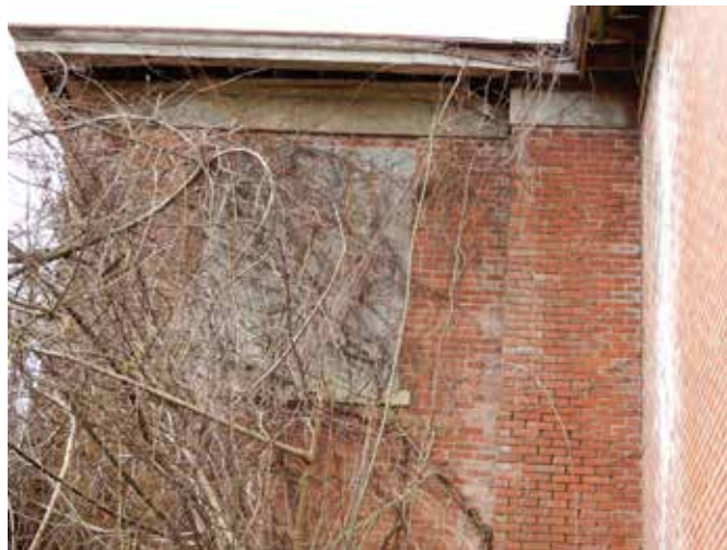
View of deteriorated roof soffit, invasive vines and mortar deterioration due to lack of gutters and downspouts.
