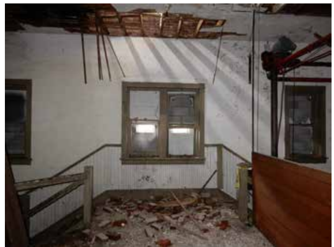
View at top of stairs showing open roof, plaster damage and original windows.
