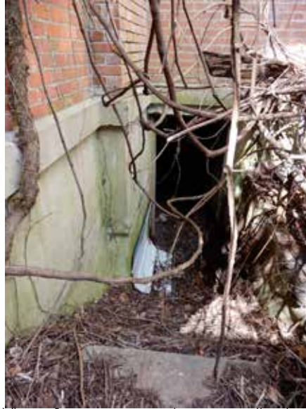
View of open access to basement allowing water and debris infiltration.
